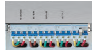
Front termination of breakers for easy access
