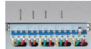
Front termination of breakers for easy access
